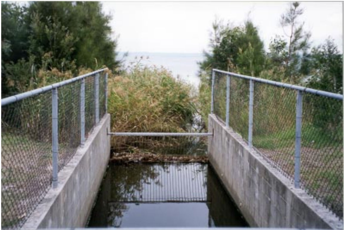
Stormwater drain at Canton Beach.
